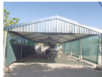
A steel structure like this has been donated to a church in Zambia.
